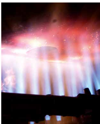
Pipe Heating Pipe Heating
